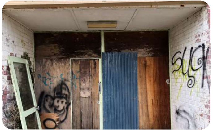
Plate 40 Site Image of current neglect
