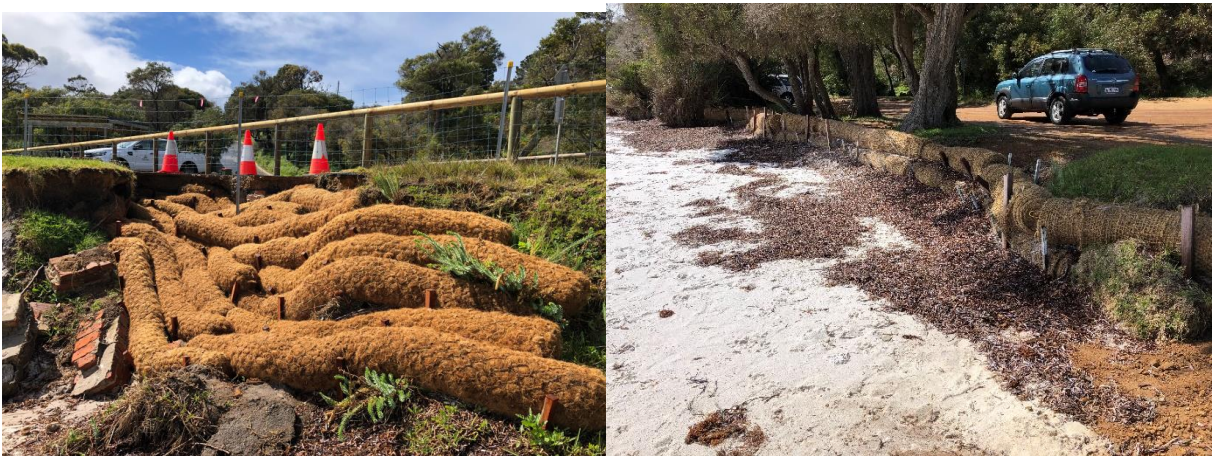
Figure 3.13 Coir Logs Installed by the City of Albany in 2021 to Combat Erosion
