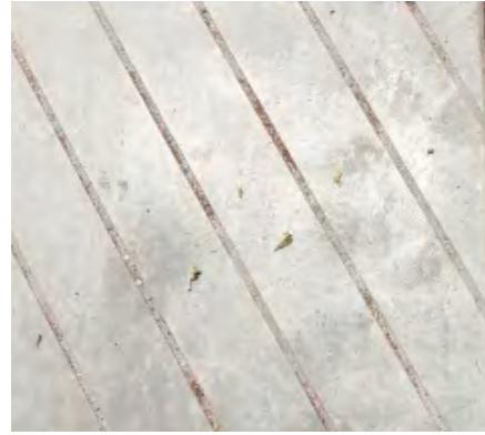
Foyer connection In-situ concrete Colour - GP Grey Finish -Wood float and saw cut
