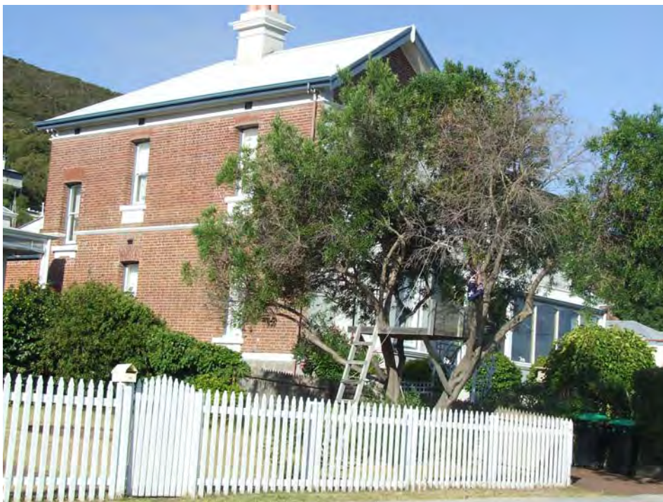
South-west elevation showing face brick to this side of the building [H Munt 2018]
