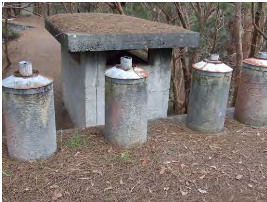
Engine Exhausts [City of Albany, 2010]
