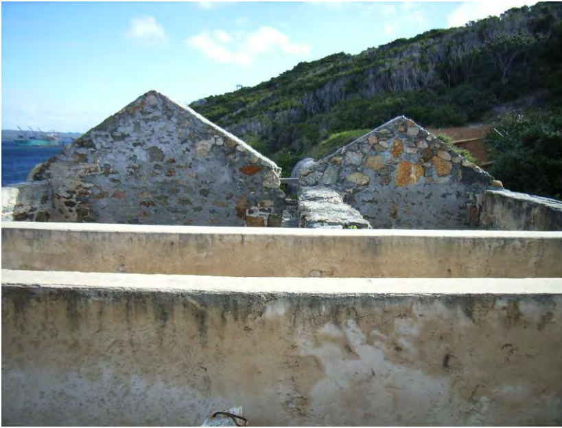
Looking over the top showing former gables and cement capping on top of wall plate [H Munt 2009]
