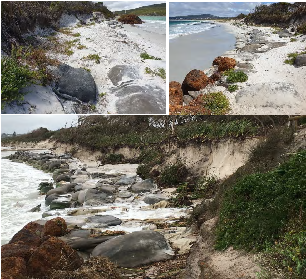
Figure 28: Erosion and state of the beach and GSC trial groynes and GSC revetment at Emu Beach, taken 26 th February 2020 (top) and August 2020 (bottom).
