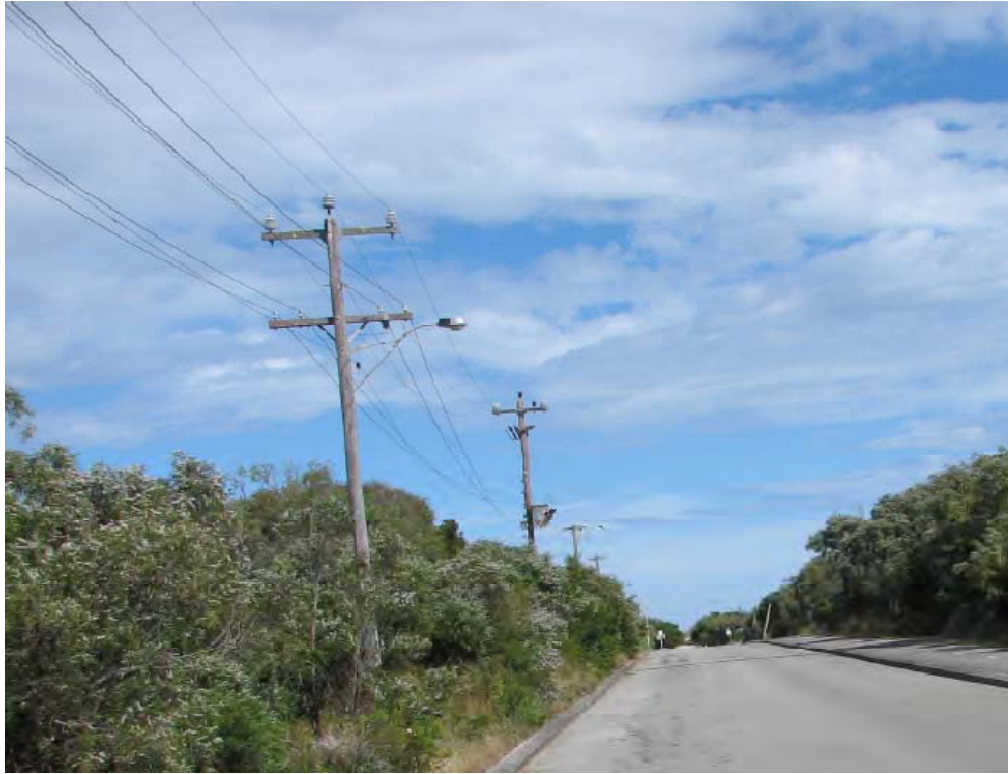
Plate 10 – Aerial power lines in Emu Point Drive
