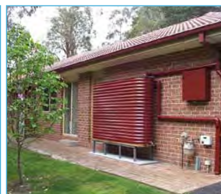
Slimline domestic rainwater tank
