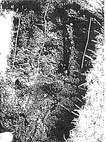
Minor seepage at 600 mm
