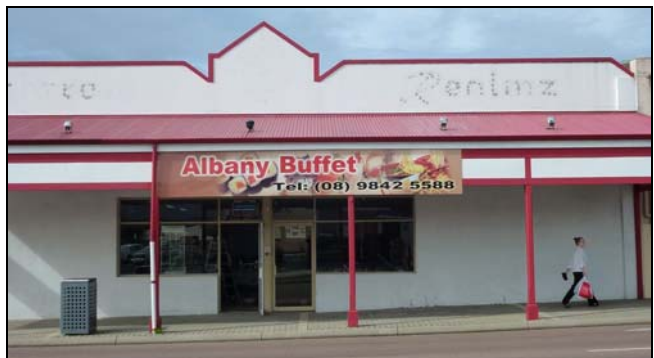
Sign design unrelated to fascia of awning.
