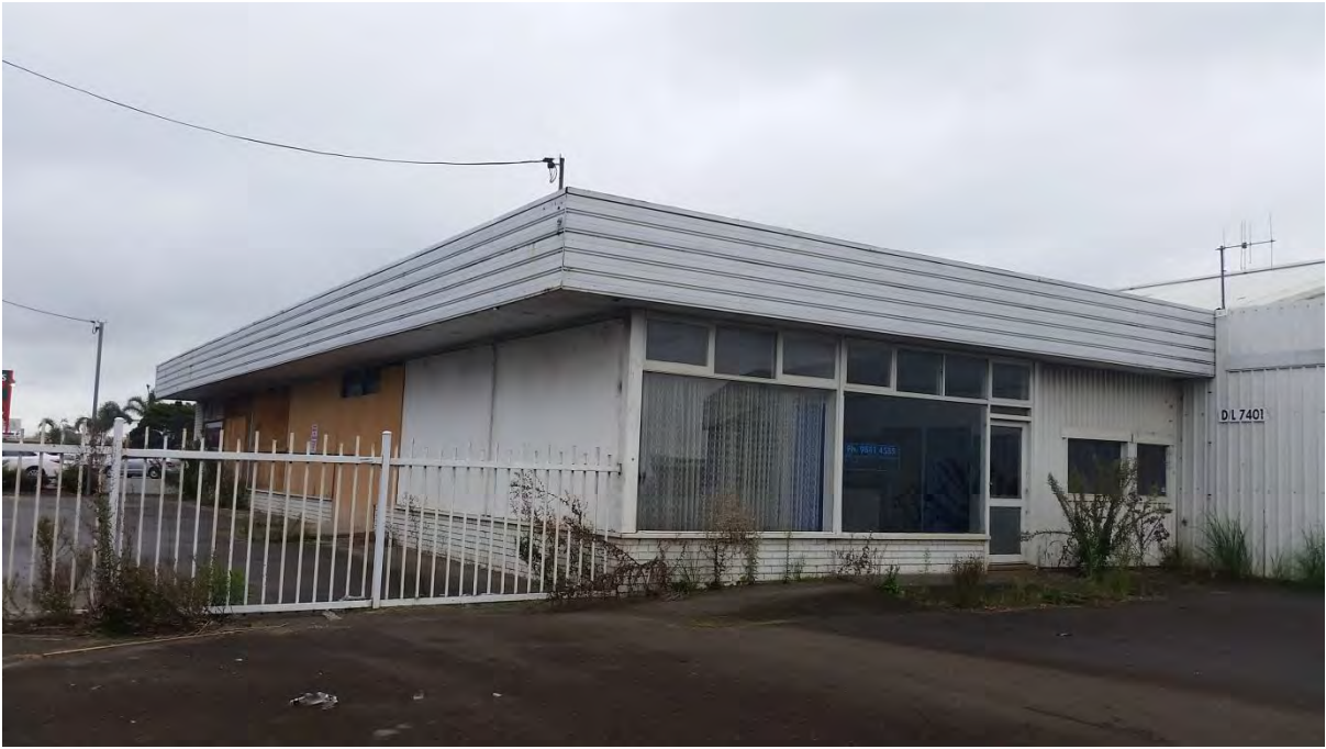
Photograph 1: Existing derelict improvements on the subject site.
