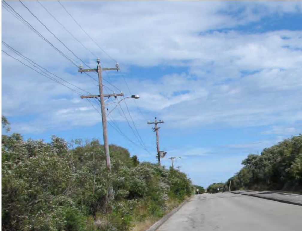
Plate 10 – Aerial power lines in Emu Point Drive
