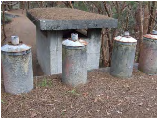
Engine Exhausts [City of Albany, 2010]
