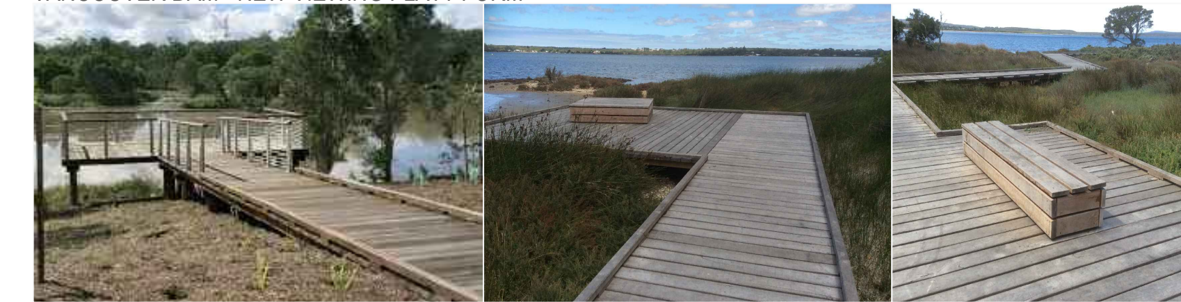
TIMBER DECKED VIEWING PLATFORM WITH TIMBER SEAT AND A TIMBER BOARD WALK FORMING THE TRANSITION TO NEW LIMESTONE PATHWAY
