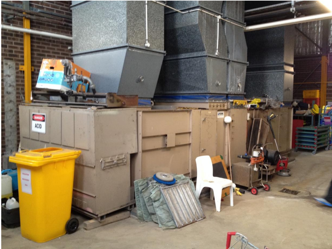
Figure 1 – Trane Lap Pool Air Handling Unit
