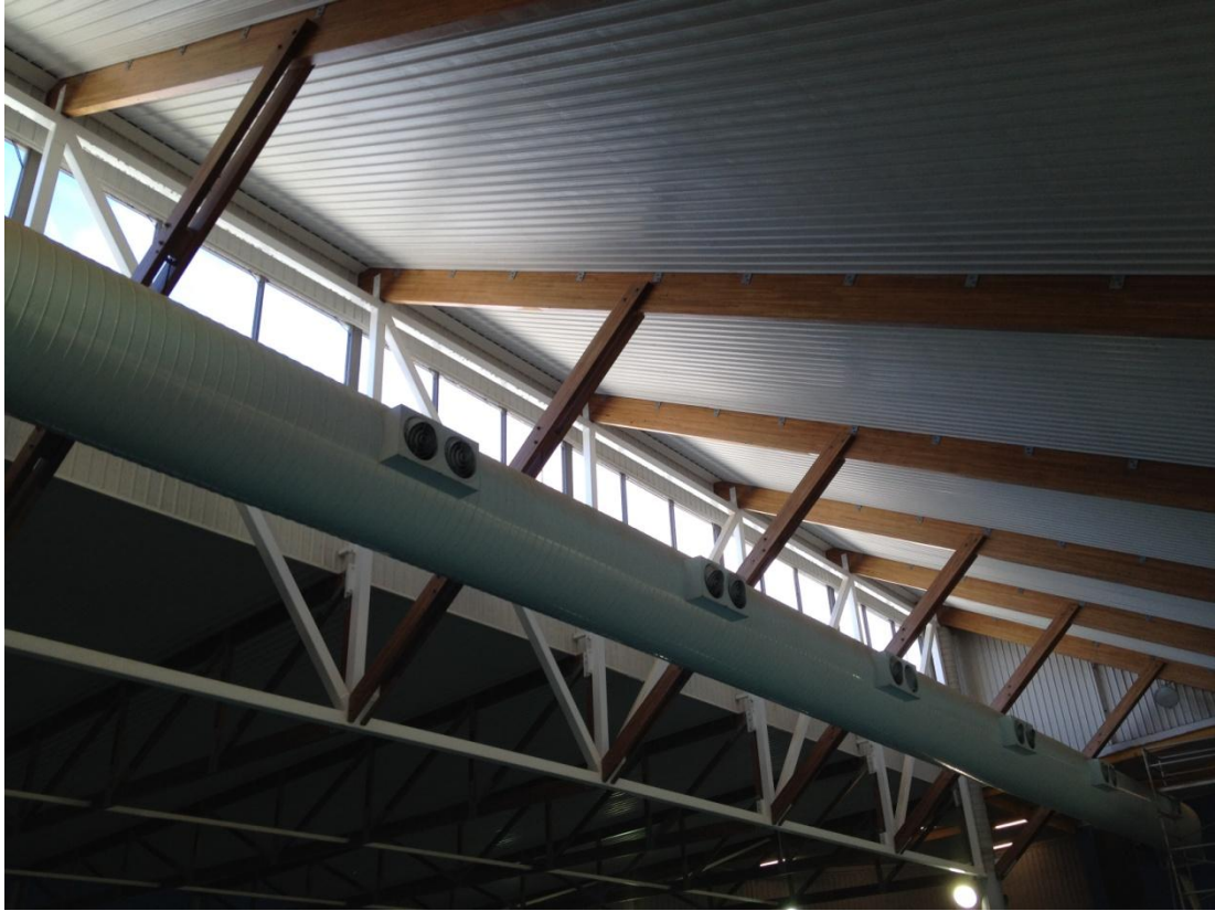
Figure 11 - Supply Air Spiral Duct
