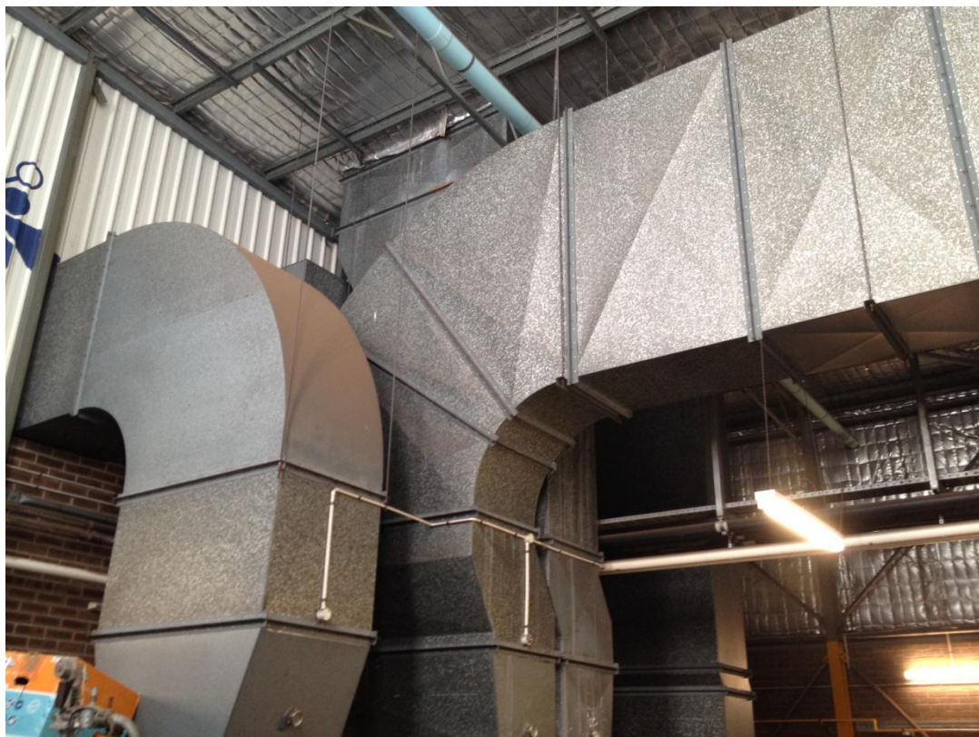
Figure 2 - Plant Room Duct Work
