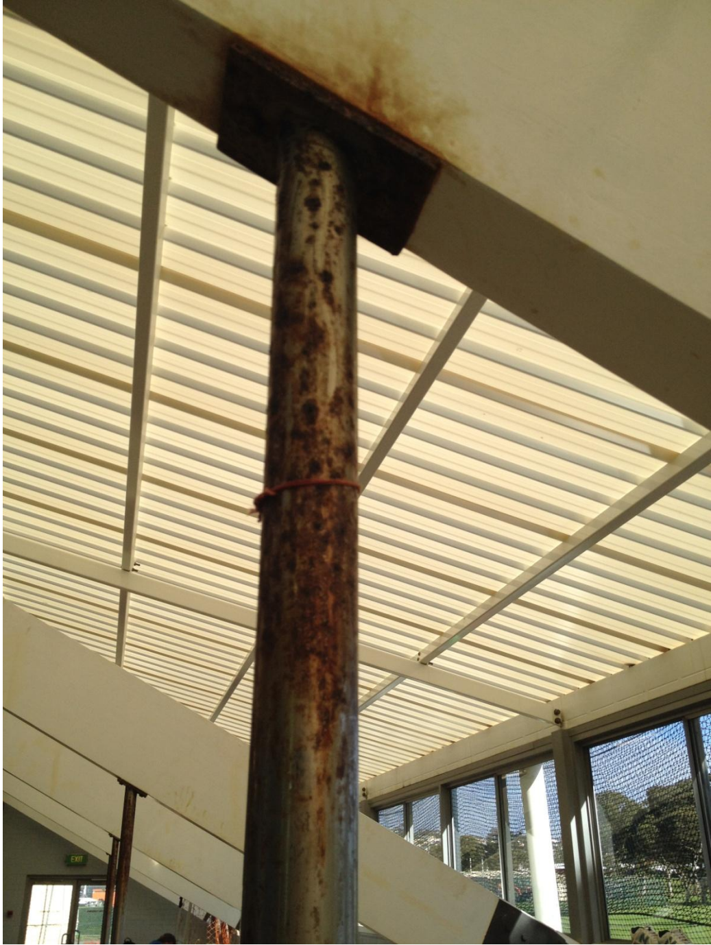
Figure 13 - Corrosion to Stainless Steel Bollards
