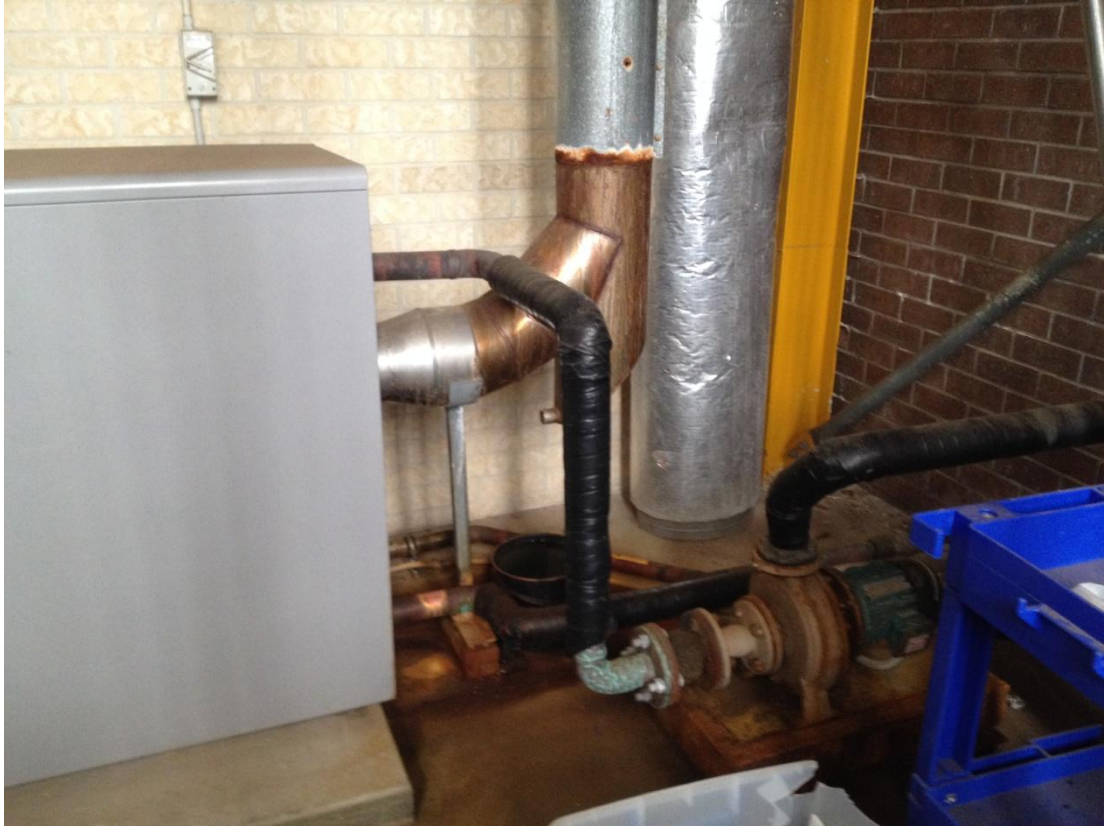
Figure 5 - Boiler Flue & Pump
