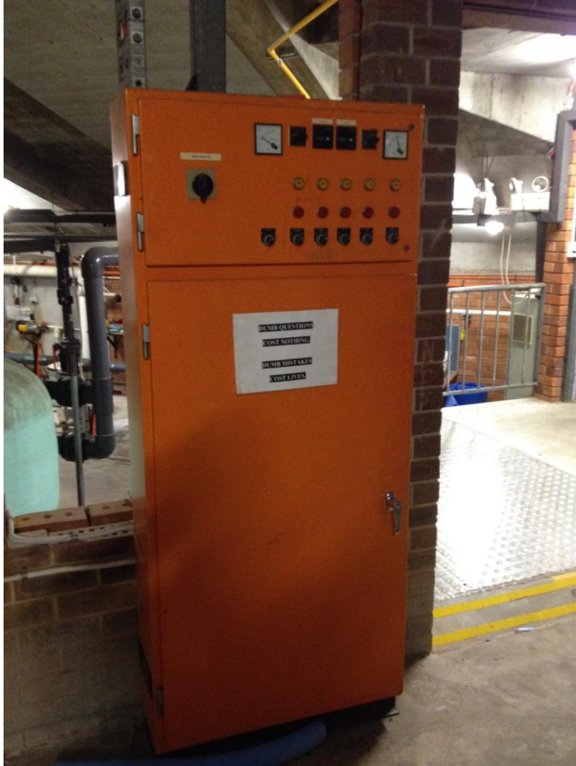
Figure 9 - Mechanical Services Switchboard
