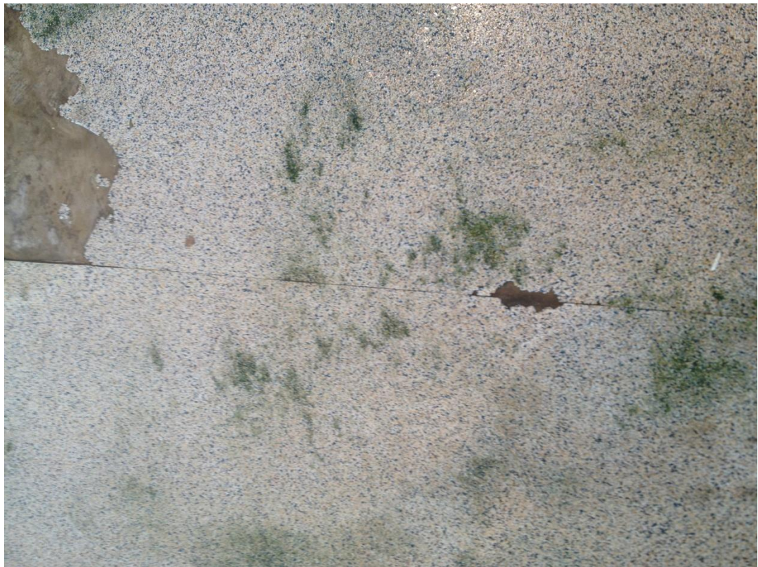
Figure 12 - Degradation of Concourse Flooring Material
