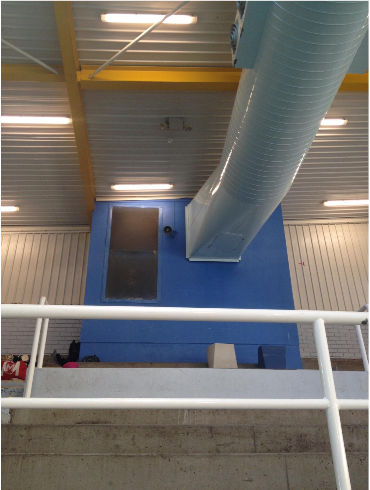
Figure 10 - Spiral Supply Air Duct and Exhaust Air Intake
