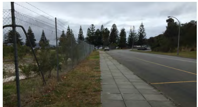
Figure 10: Poor Condition of Pedestrian Infrastructure Adjacent to MBAC
